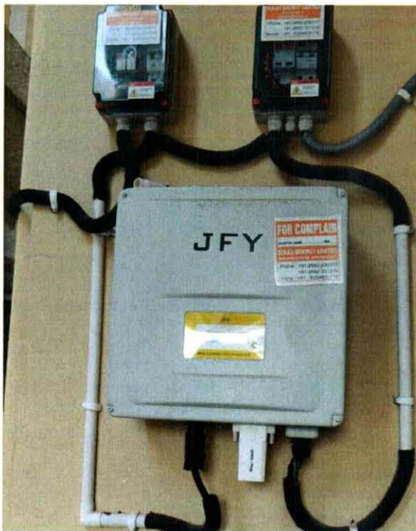
B: cables in conduits and neatly routed
